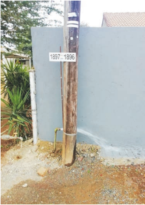
A significant amount of potable water was wasted.
